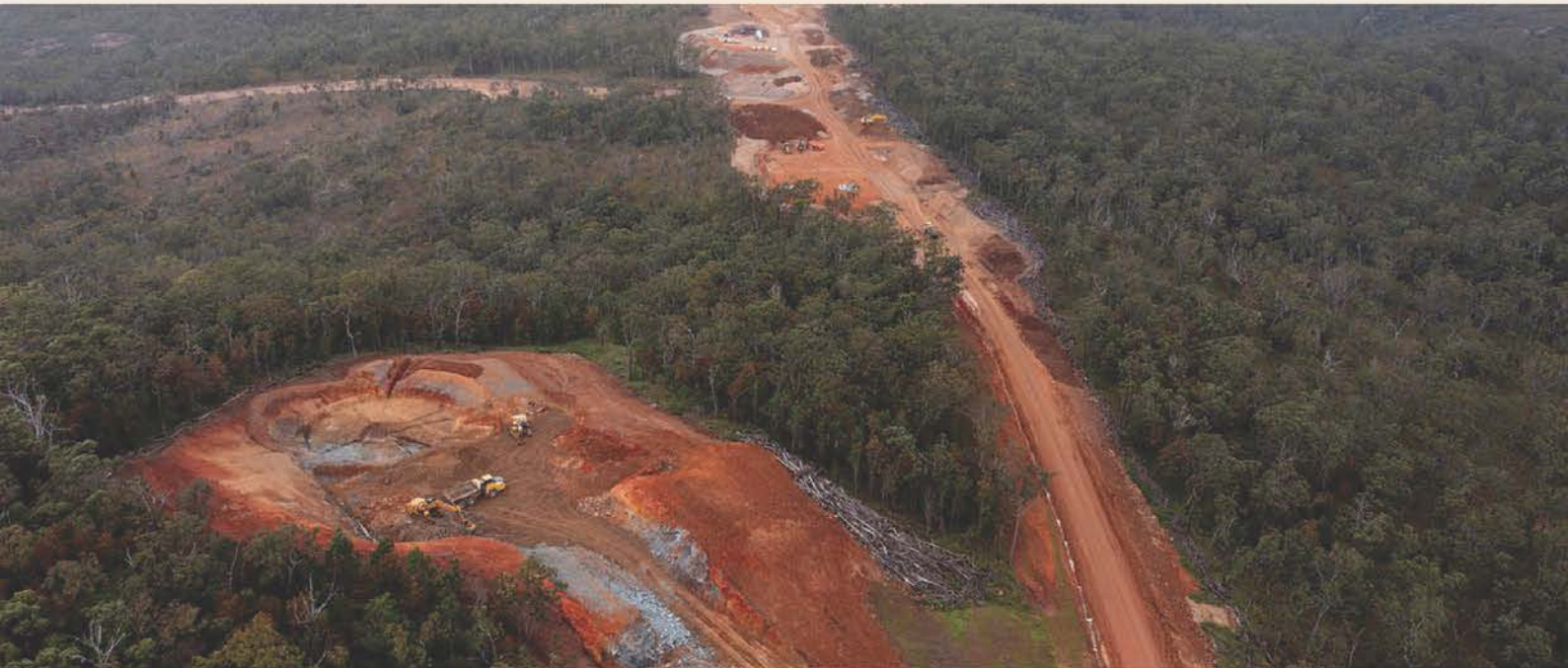
Photo by Steven Nowakowski - Example of clearing during a Wind Farm construction in Far North Queensland
