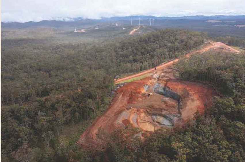
Photo by Steven Nowakowski - Example of clearing during a Wind Farm construction in Far North Queensland
