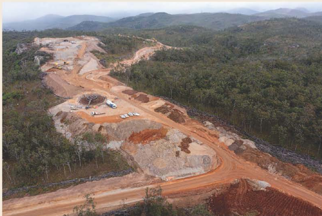
Photo by Steven Nowakowski - Example of clearing during a Wind Farm construction in Far North Queensland
